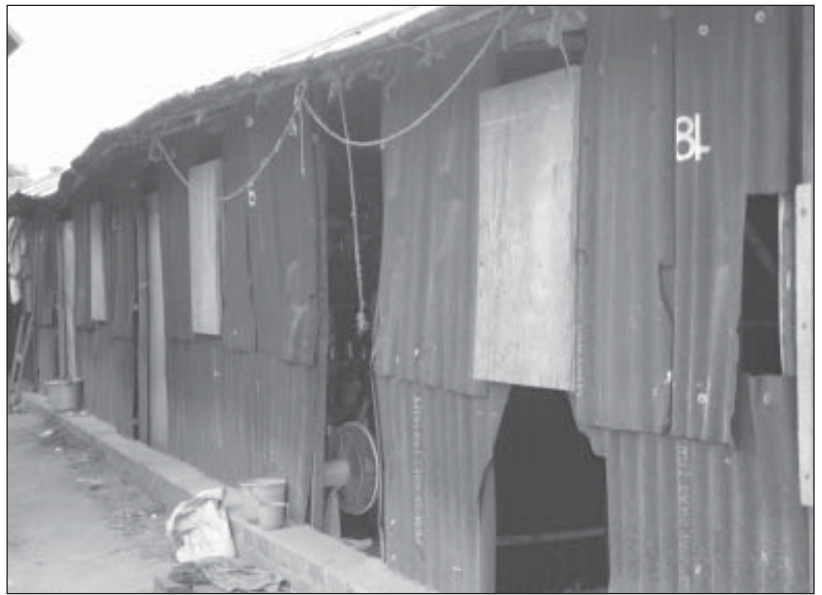
Temporary line housing built of tar sheets in Tamil Nadu clearly showing the inadequacy and poor durability of the material used.
