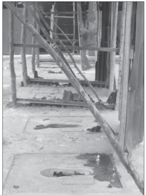
Unusable toilets in Akkaraipettai, Nagapattinam.
