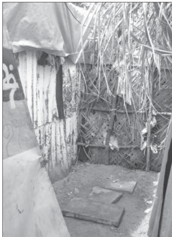
Space in between two shelters being used by women for bathing, due to lack of bathrooms for women in the temporary housing settlement of Pudu Nemellikuppam, Cuddalore, Tamil Nadu
