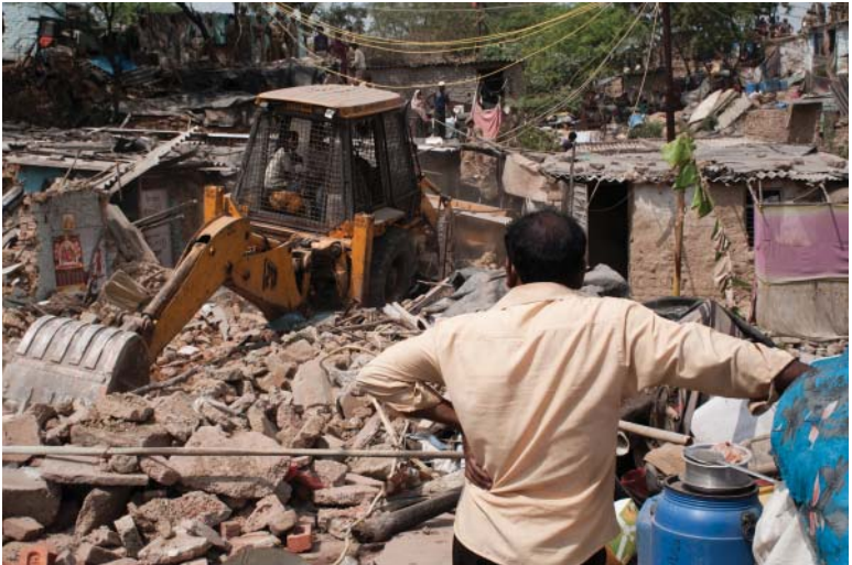
A resident watching his house being demolished. No relocation has been provided by the Government
