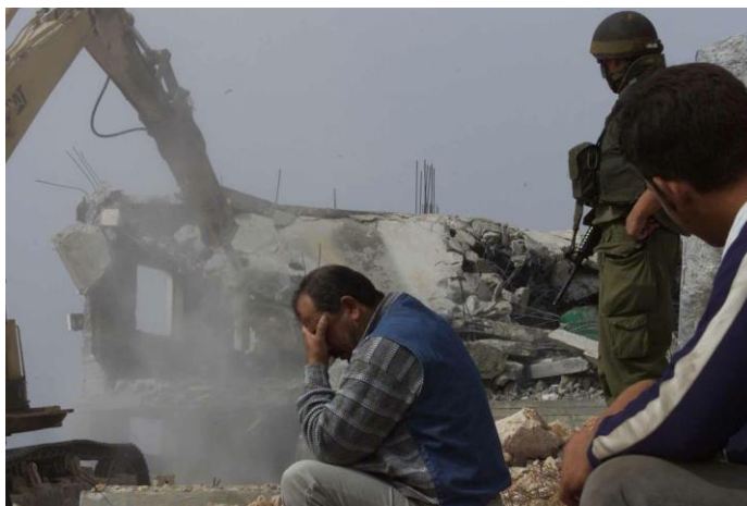
Israel demolition of Jerusalemite Palestinian homes, in Beit Hanina, 29 October 2013. Source: ECCP.
